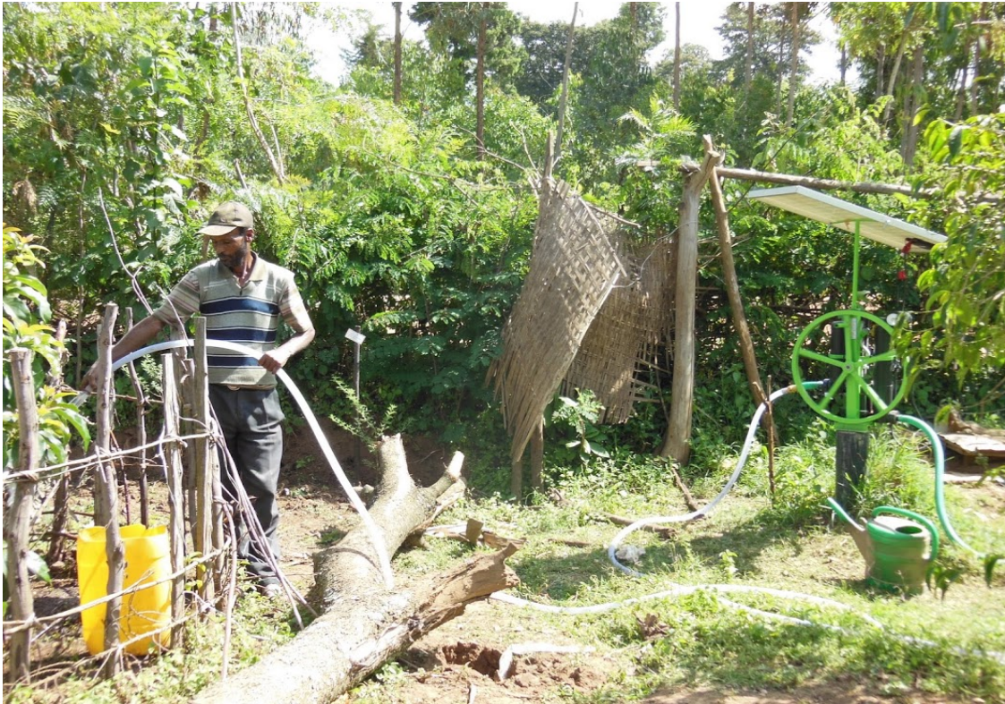
Solar pump system
