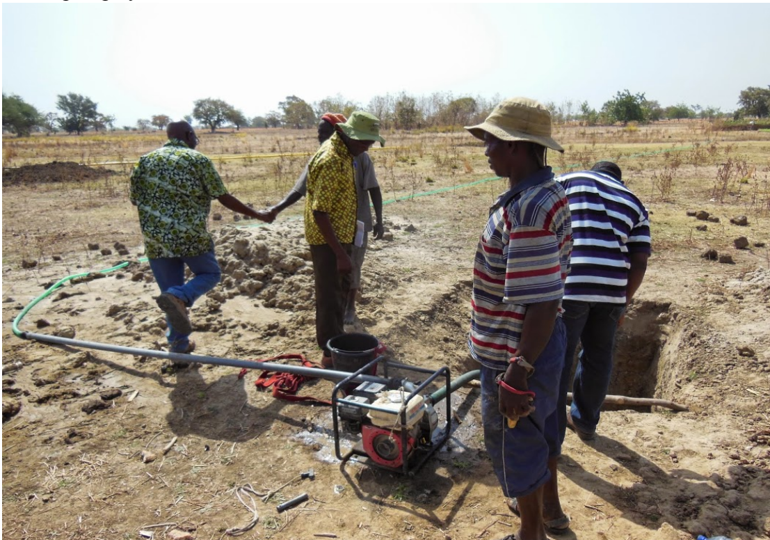
Motor pump system
